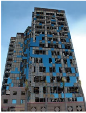
The Kathleen C. Wright Building will have approximately 1,000 windows replaced during the site's Hurricane Wilma-related repair project.
